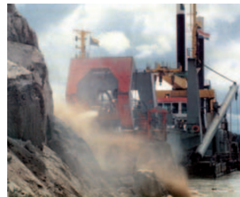
Boskalis will bring in the latest technology and equipment, and employ up to 150 local workers on the project
